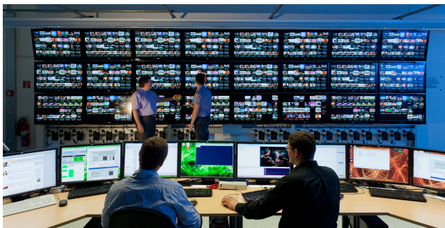
Photo: Kabel Deutschland - Digital TV-Broadcasting at the KD Playout Center in Kirchheim
