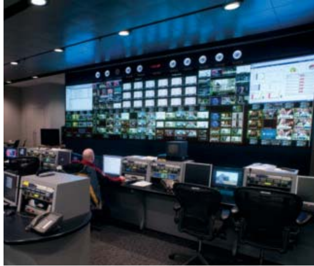
Rogers Communications Signal Monitoring Facility
