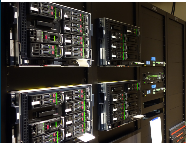
Mediator Playtime running on blade servers
