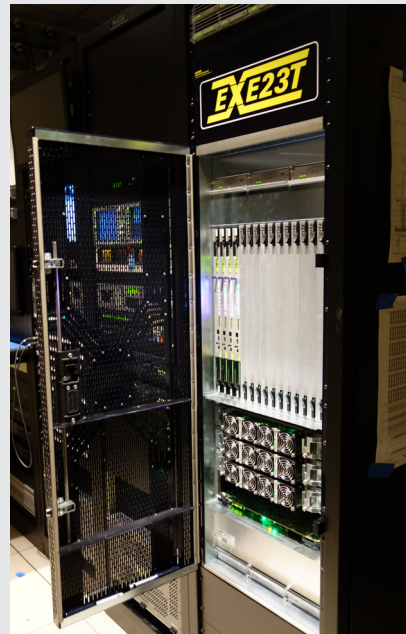
EXE IP Switch Fabric - Inside
